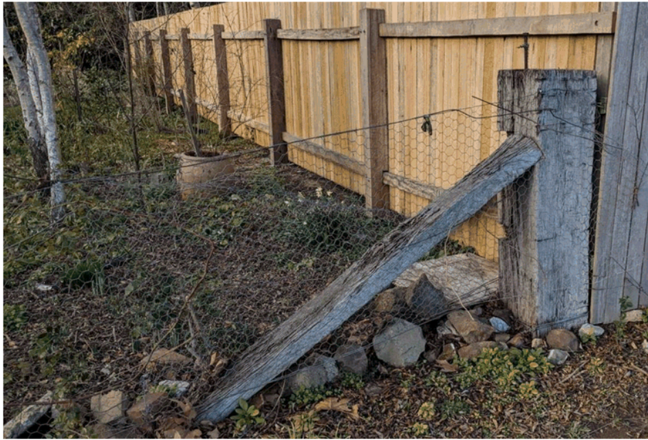
A specific view of the corner post and strainer. This is a distinctive feature of the site and should be retained.
